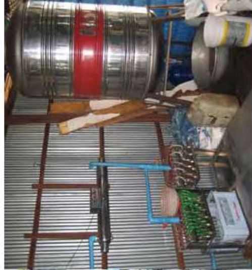
6/ UV water treatment, Chhnok Trou
